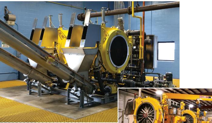
Municipal Water & WWT Plants Madisonville, Kentucky
